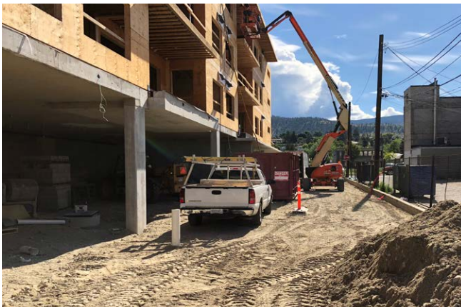
◀ Photo of a BC Housing affordable housing project construction site in Penticton, BC.
