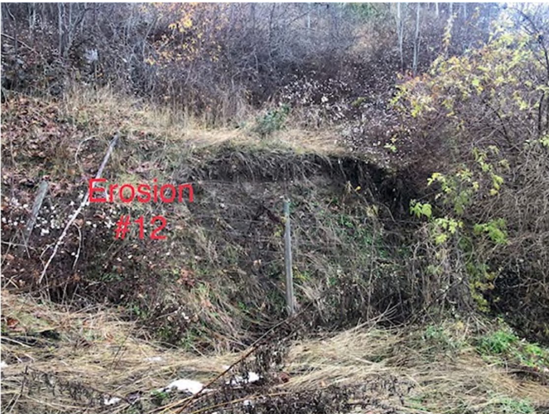
Photos showing the erosion starting to happen at the bottom of the ridge
