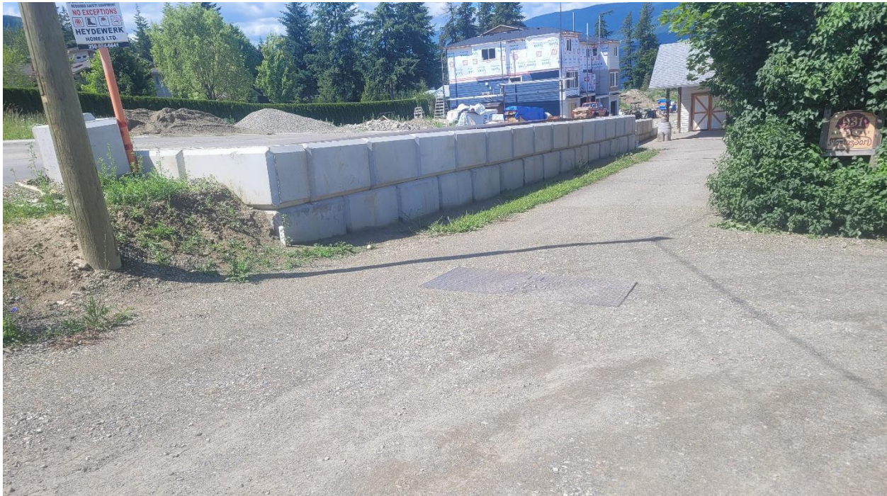
Photo 1: Lock-Block retaining wall along property line between 981 12 Street NE and 931 12 Street NE. Development Permit application proposes to install a privacy fence along the top of the retaining wall.
